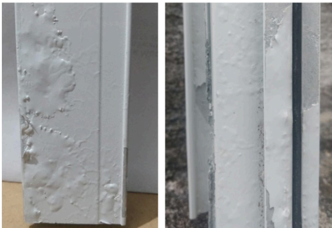
Figure 2 – Filiform corrosion in aluminum profiles
