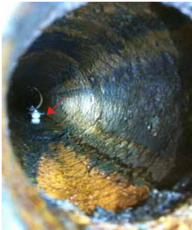
Figure 4 - Internal view of the test section showing the corrosion product removal. Source: Authors.
