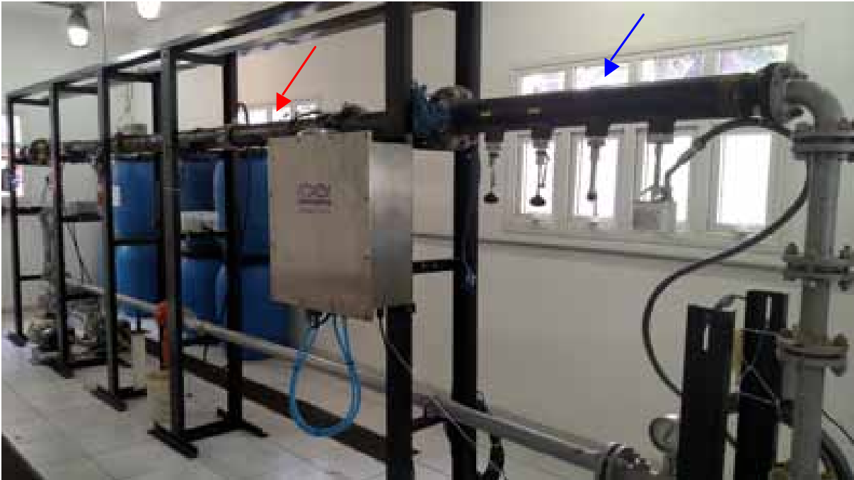
Figure 1 - Corrosion loop used to evaluate non-intrusive techniques. Source: Authors.
